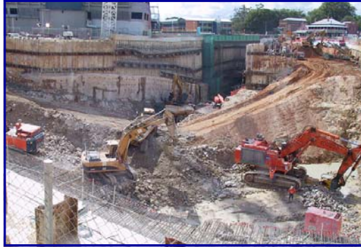
The Kedron Hotel (top right) is dwarfed by the huge excavations required for these Airport Link Tunnel connections (R S-W)
