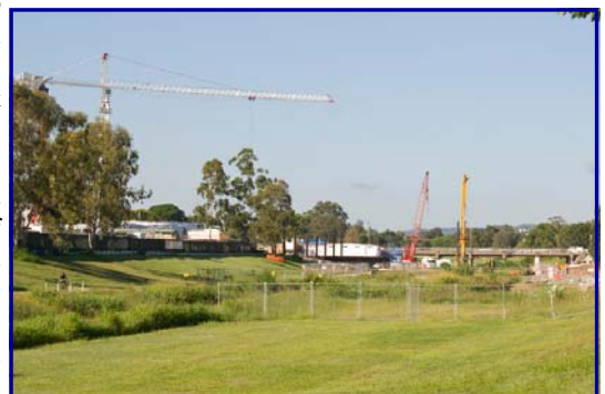
Cranes work to complete the huge Gympie road and connecting bridge works over the Brook at Kedron
