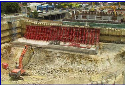
Massive formworks being prepared for the Gympie Road and connecting laneways to cross the Brook at Kedron (R S-W)
